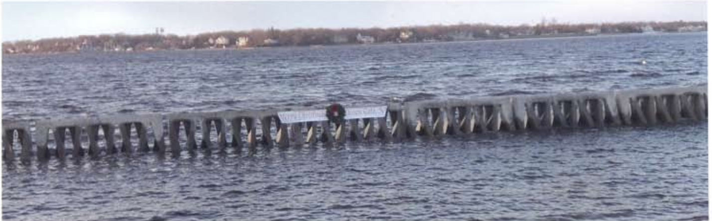
The Army Corp of Engineers required that the prisms be installed only between July 1 and December 31, to avoid disrupting the winter flounder run that takes place off the New Jersey coast.
